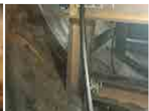
MIV Blade Seal before repair
