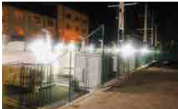
1MW generators at Kolonnawa site -02
