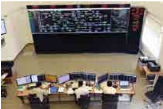
Figure Tr-3: System Control Centre
