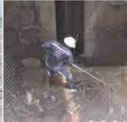
Cleaning the Intake control system
