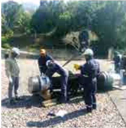
New CT before installation
