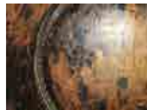
MIV Blade at close position before repair
