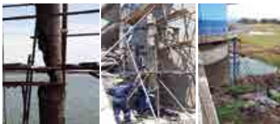
Corroded steel pipe
