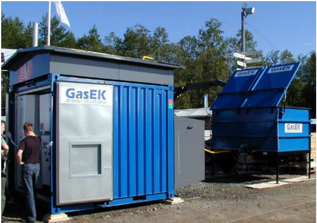
The GasEK small scale CHP-plant is a brand new Finnish innovation, which can gasify wood chips of under 40% moisture content. Total output of the plant is 90 or 150 kW, which includes about 33% electricity. (Photo: Timo Lötjönen, MTT)
