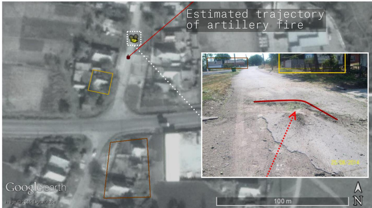
Figure 23. Geolocation of the artillery crater from @tombreadley on Twitter 100 (position: 47.124413, 38.069940). The trajectory of the artillery crater is identified on the map with a solid red line. Damage to a house on this street from this attack is shown in video 26-8 101 .
