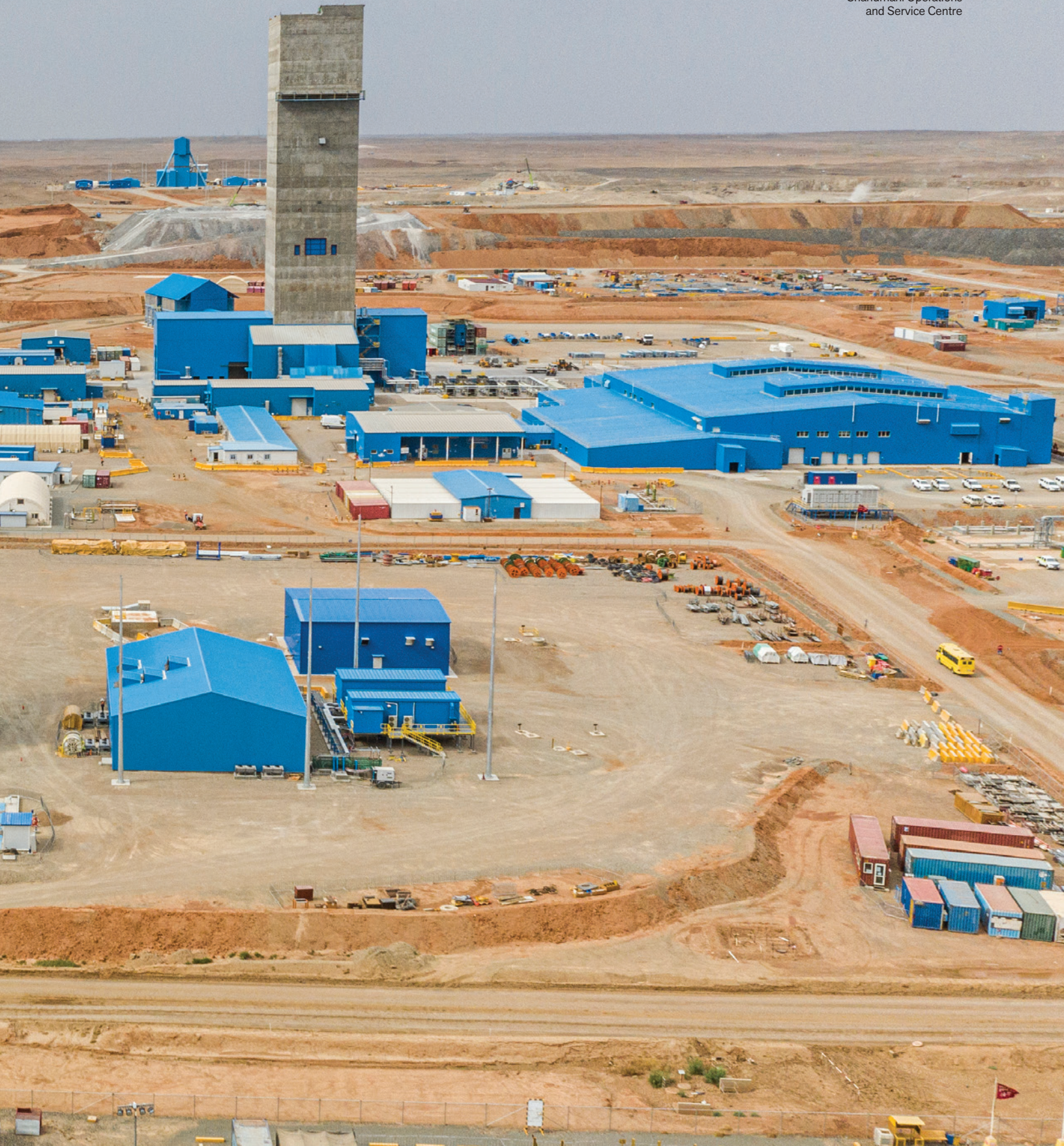
Underground Mine Shaft Facilities and Chandmani Operations and Service Centre
