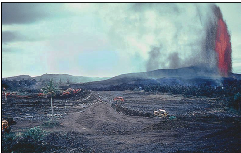
Figure 5. Photograph showing bulldozers constructing a lava flow barrier in Kapoho in January 1960. Note the advancing front of an ‘a‘ā flow between the lava fountain and the trees at left. Date of photograph and photographer unknown.
