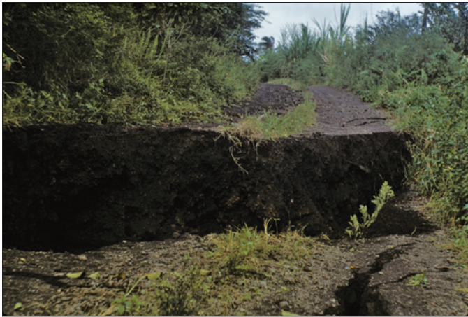
Figure 13. Photograph showing earthquake offset of Old Railroad Bed Road along the Koa'e Fault north of the village of Kapoho, prior to a Kīlauea eruption. The road is vertically offset about 1.5 m. The Koa'e and nearby Kapoho Faults are old structures, reactivated in April 1924 during major collapse of the Kapoho graben and again in 1960. These faults still exist and will doubtless move again (USGS photograph taken January 13, 1960, by J.P. Eaton).
