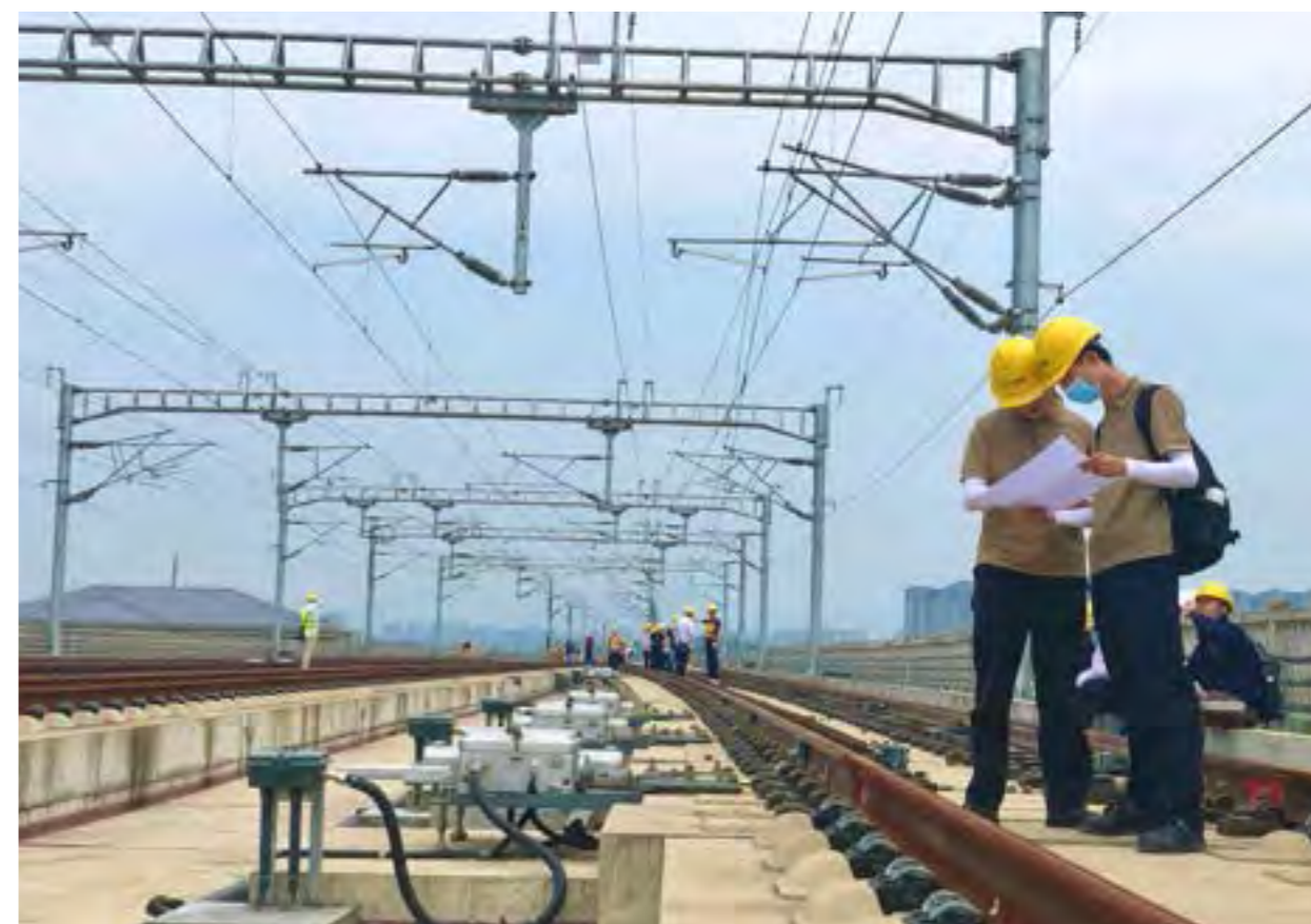
专业人员确认转辙机位置安装情况 Professionals confirm the installation location of the switch machine
