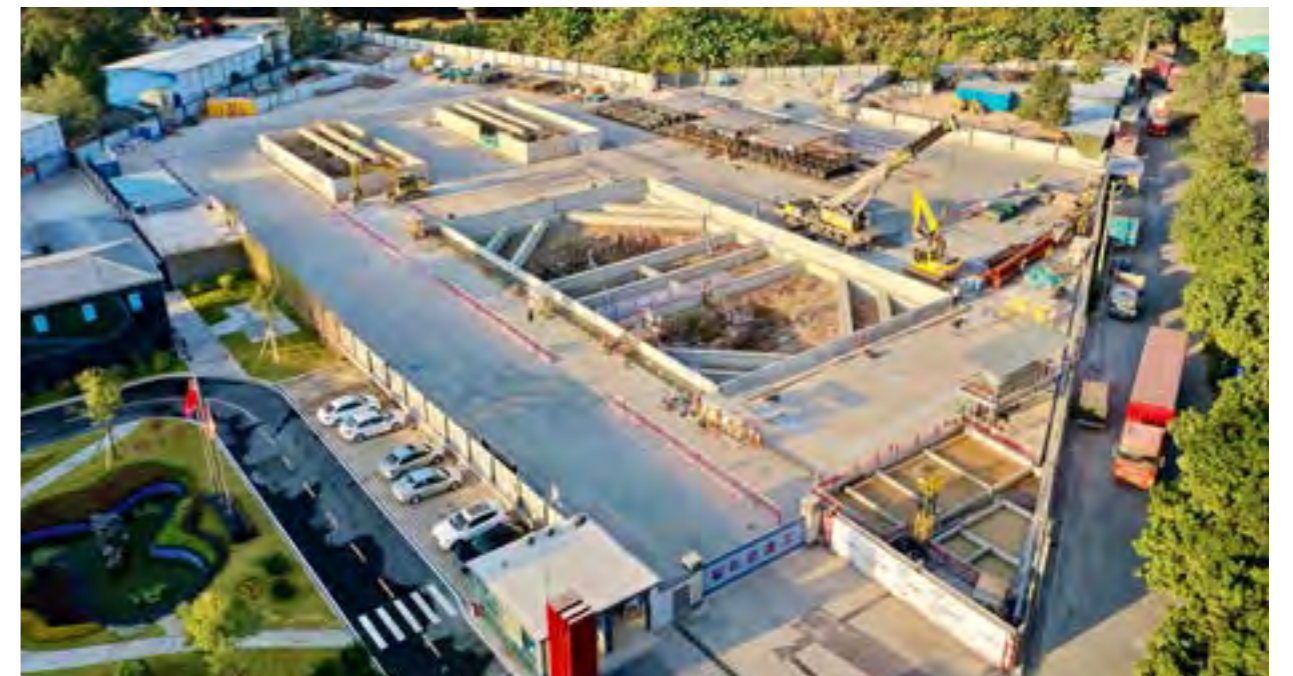
五号线东延段双庙区间中间风井 Intermediate air shaft of Shuangmiao Section, Eastward Extension, Line 5
