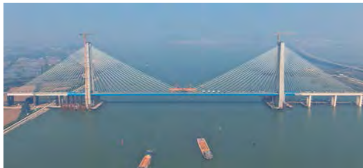
龙穴南水道特大桥胜利合龙 Successful Closure of Longxue Nanshuidao Grand Bridge
