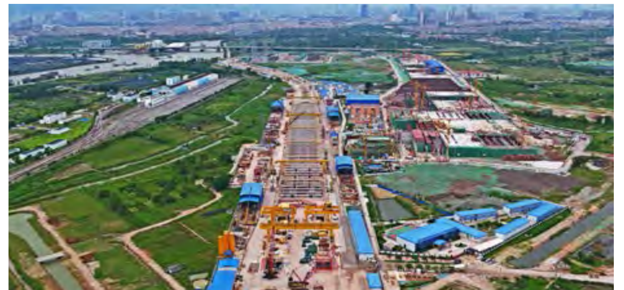
二十二号线陈头岗站及陈头岗停车场出入场线 Entrance and exit section lines of Chentougang Parking Lot and Chentougang Station of Line 22
