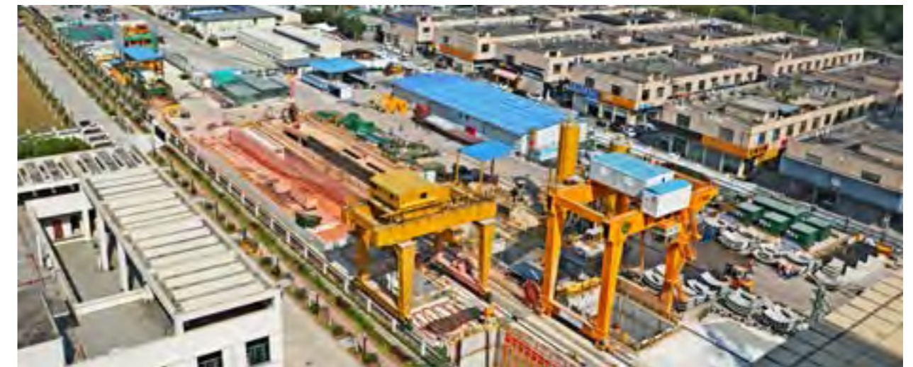
十四号线二期彭边至嘉禾望岗区间台车吊装 Vehicle hoisting at Pengbian– Jiahewanggang section, Phase-II of Line 14
