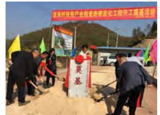
为流洞村产业园道路奠基 Laying the Foundation for the Liudong Village Industrial Park Road
