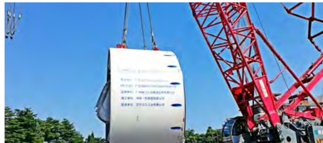
七号线西延段“奋进号”盾构吊装 Hoisting of "Endeavor" Shield Tunneling Machine for Westward Extension of Line 7
