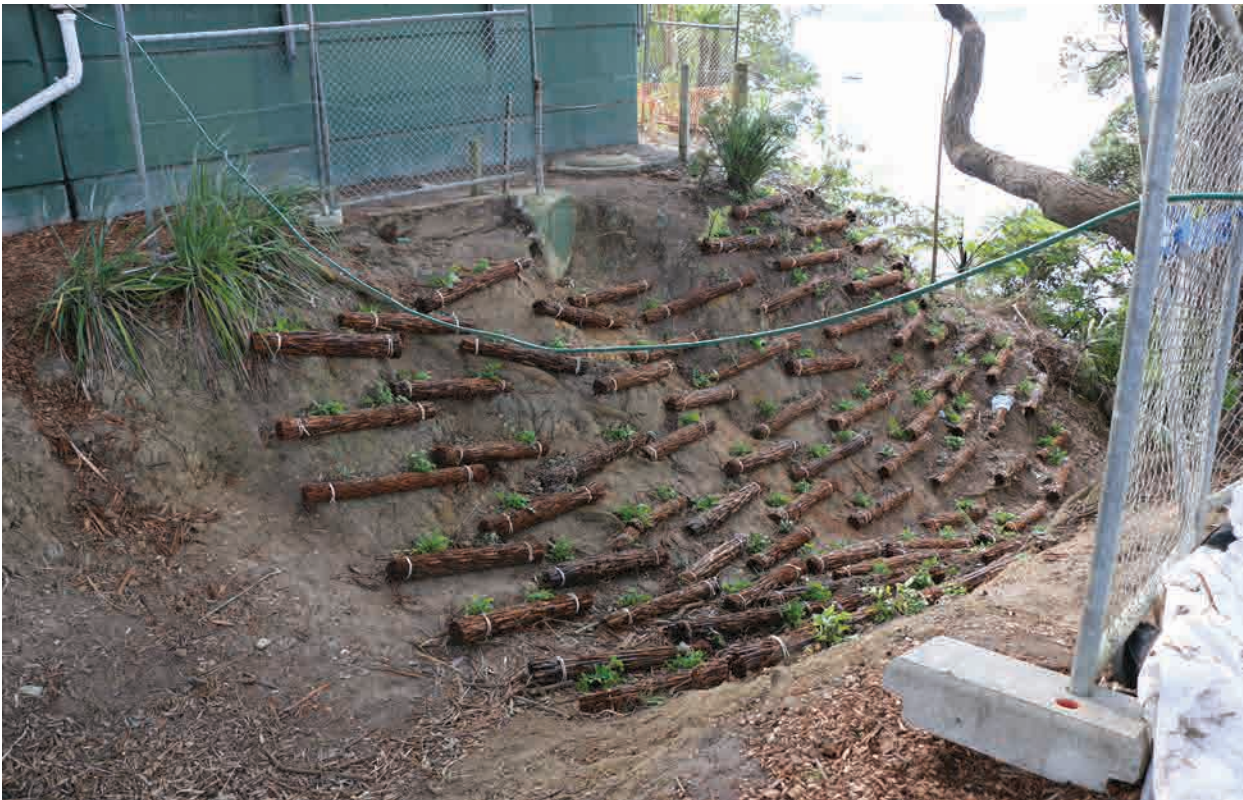
Figure 17. Ponga held in place in ditch prior to replacement foot bridge being installed.
