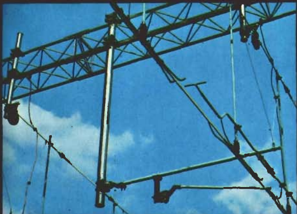
Overhead wiring pattern.
