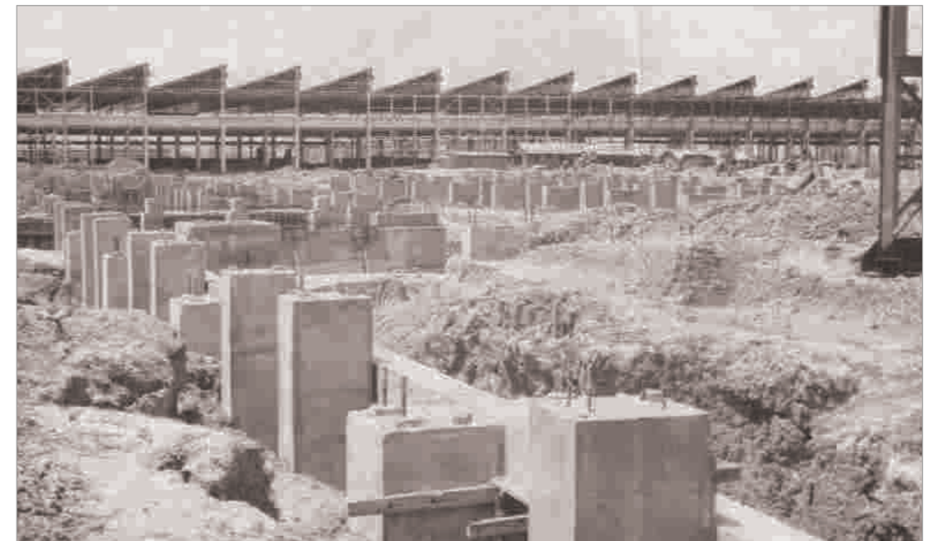
1965: A view of the construction site of Bloom Cast Mill at Alloy Steels Plant, Durgapur
