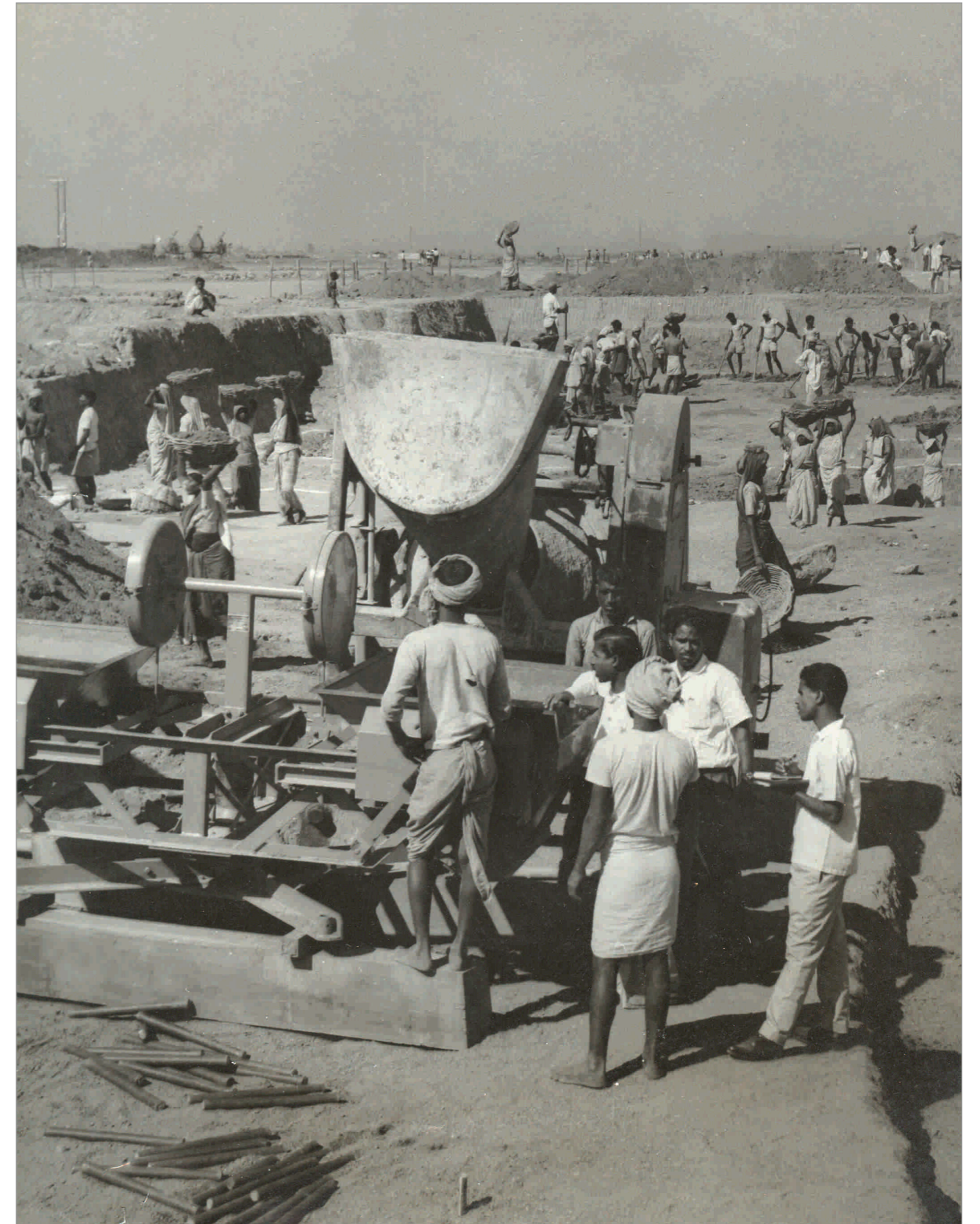
November 27, 1967: Levelling work in progress at the site of Bokaro Steel Plant
