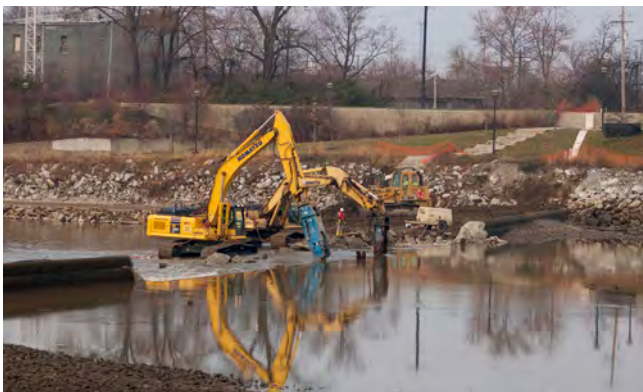
The Main Street Dam was breached in November 2013.
