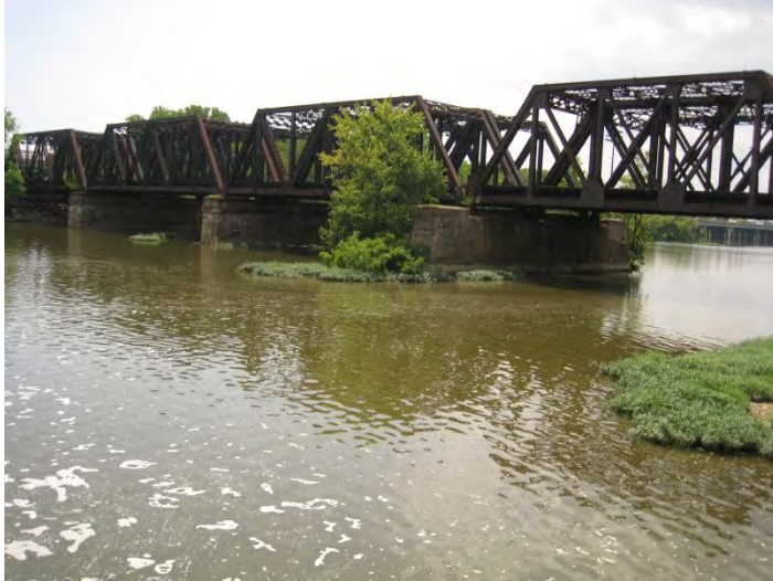
Photo 8-1. NS/CSX Bridge showing aggradation at pier
