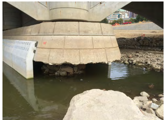
Skirting the pier caps proves difficult to angle and curvature.
