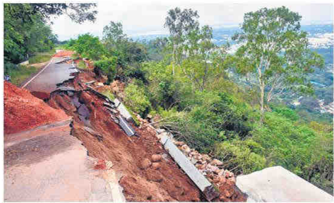
PLANS FOR TREKKING? NOT NOW Chamundi hill road in Mysuru, which caved in following heavy rains, seen damaged further on the weekend | UDAYSANKAR S
