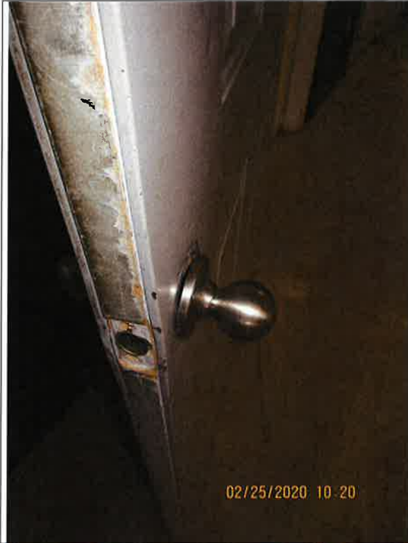
Small lounge Broken doorknob and missing door plate
