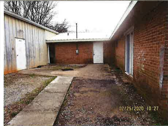
School building entry Rundown, unsafe and inaccessible entrance
