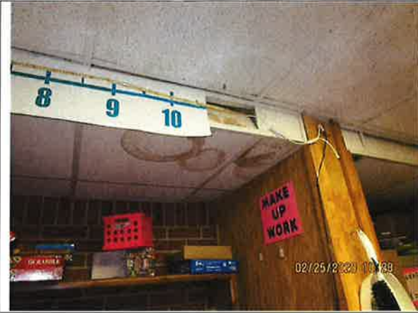
Water damage in classroom ceiling
