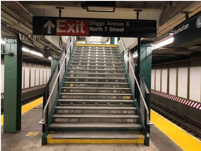
View looking west at the new P6 platform stair to the Driggs Avenue mezzanine at the Bedford Avenue station.
