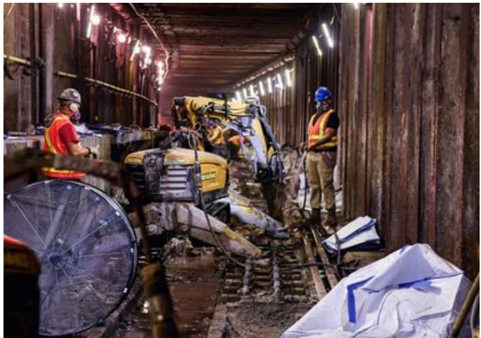
Photo above and the first two on the next page show some views of the track reconstruction work on the upper level of the Archer Avenue Line all taken on September 30. Marc A. Hermann / MTA New York City Transit photographs
