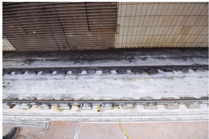
View of Type VIII track structure at Sutphin Boulevard/Archer Avenue station before reconstruction on September 30. Marc A. Hermann / MTA New York City Transit photograph
