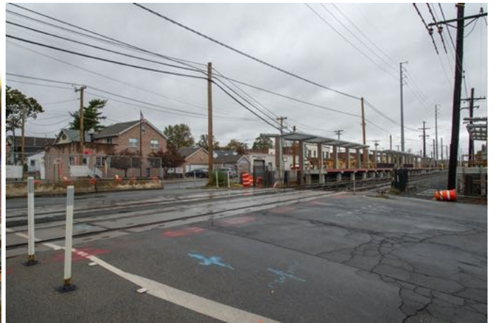
One week later, on October 30, with South 12th Street closed off. Only the crossing gate mechanisms and flashers have been removed. Jeff Erlitz photograph
