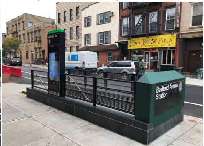
The new stair on the southeast corner of Driggs Avenue and North 7th Street, oriented south along Driggs Avenue. Note the vertical digital information display, the stair enclosure, and railing are all in a style similar to what has been installed at stations rehabilitated under the Enhanced Station Initiative.
