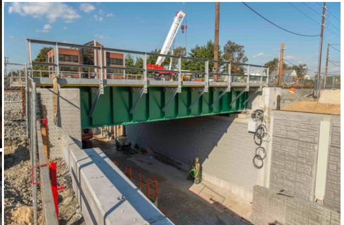
The new three-track bridge carrying the Main Line over School Street, on the Westbury/New Cassel border, as seen on October 9.
