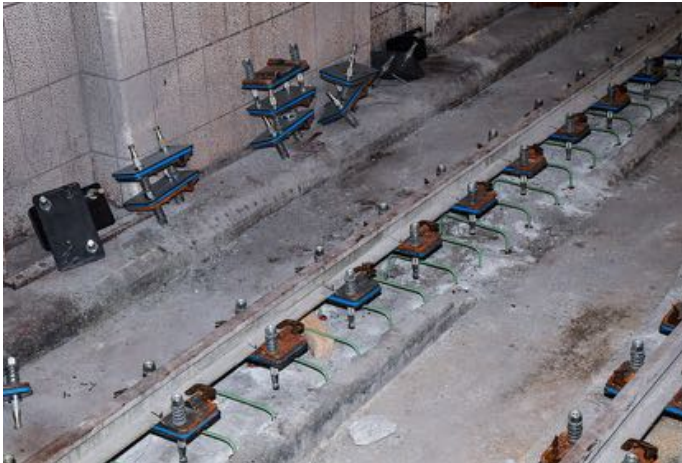
Rebuilt track structure prior to the pouring of concrete in the Sutphin Boulevard station.
