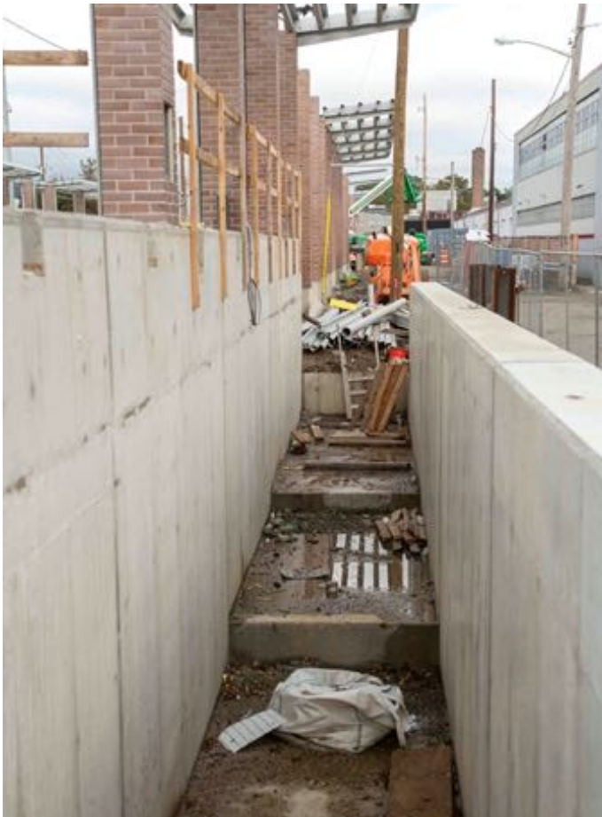
View looking east on October 23 at the pedestrian underpass which is under construction on the south side of the right-of-way, just east of South 12th Street in New Hyde Park.
