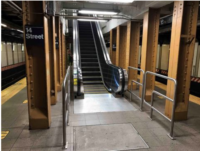
On the Canarsie Line platform at the 14th Street-Union Square station, this view is looking east at the bottom landing of the new escalator leading up to the east upper mezzanine adjacent to the IRT Lexington Avenue Line mezzanine.
