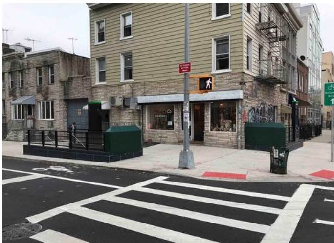
View looking northeast at the corner of Driggs Avenue and North 7th Street, with the new stair on the left, and the reconstructed 1924 stair on the right. Note that the stair enclosure ends have yet to be fitted with the station name sign and additional digital displays.
