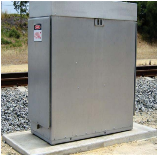
EST Electrical Supply Transformer
