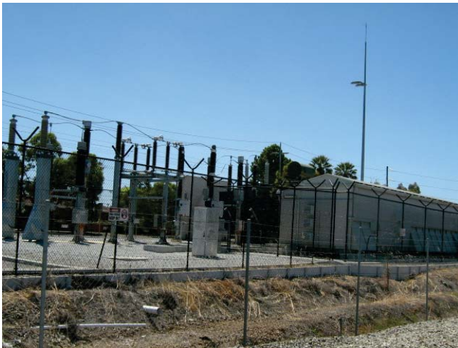
SFS Sub Feeder Station
