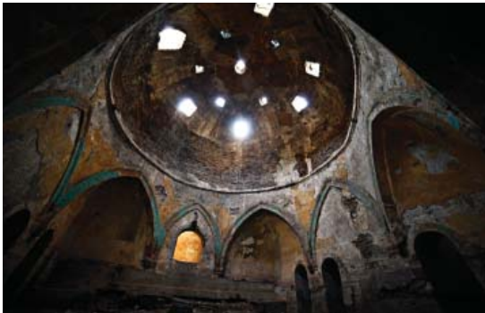
The bathhouses of Kars. Bearing a typical Byzantine style, the bathhouses were located in the lower part of the fortress, near the river. They are in a state of neglect today, filled with rubbish
