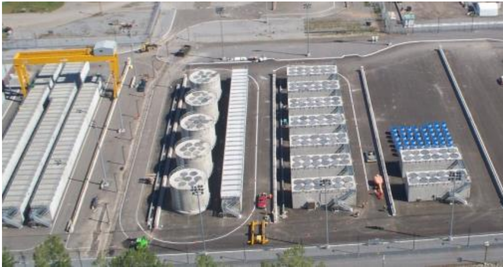
Figure 5.3: Gentilly-2 solid radioactive waste management facility
