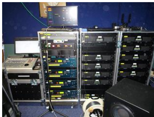
FIGURE 66 Sound equipment in the preview room
