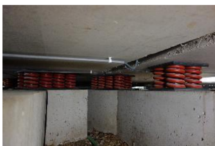
<Photo 15: Each recording area and control room at Galaxy Studios is structurally separated from each other by blocks, each of which is floated by powerful springs, providing exceptional isolation of 100.7 dB SPL between recording areas and control rooms and the world's quietest 14 dB(A) of background noise (NR value of 5). >
