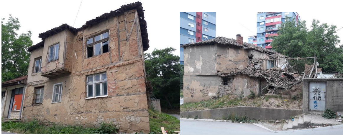
Figs. 22, 23. Old, abandoned house in North Mitrovica. Source: Fieldwork, June 2018
