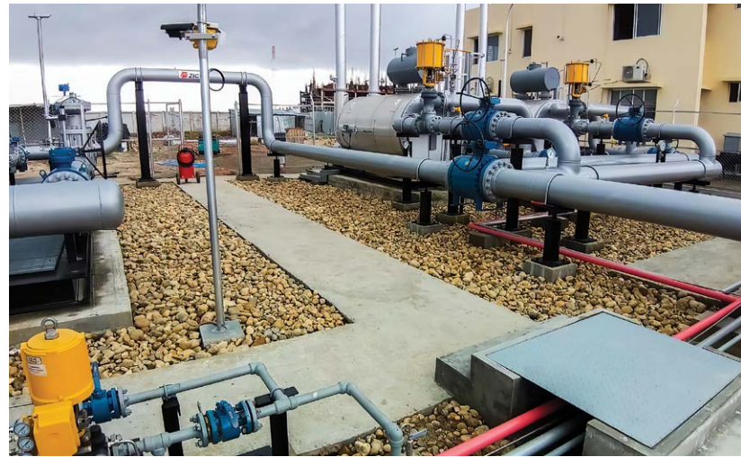
DRS-2 of KGDCL at Bangabandhu Sheikh Mujib Shilpa Nagar
