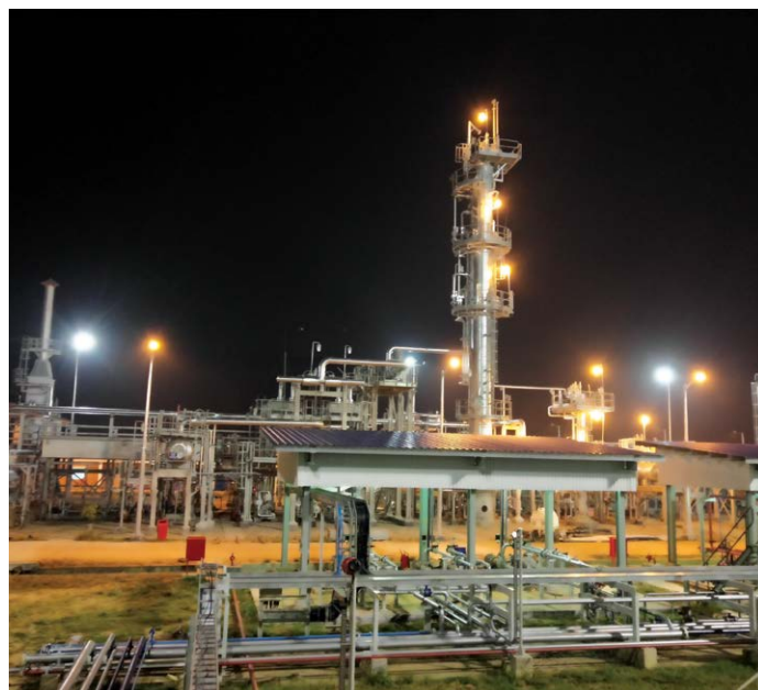
4000 BPD Condensate Fractionation Plant at Rashidpur of SGFL
