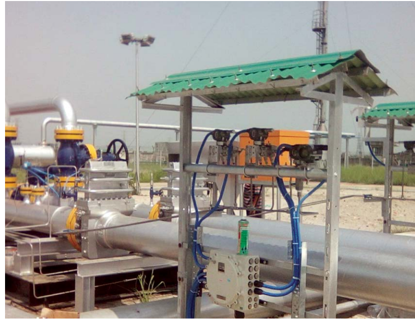
Field instrument of SCADA System of GTCL
