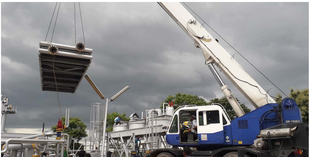
Replacement of inlet cooler of a process plant at Location-A of Titas Gas Field under BGFL
