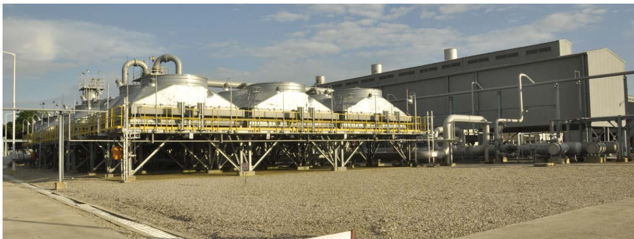
Compressor Station at Ashuganj under GTCL
