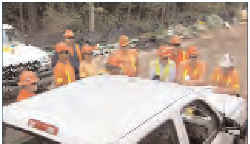
The Engineering Bridge Rehab Gang R 901 holds a safety briefing before the day's work of replacing the platform at the Thurgood Marshall BWI Airport Rail Station begins. The employee safety program stresses the importance of holding safety briefings along with individuals' involvement in reaching safety goals. (L. to R.): Ray Singleton, Mark Freyman, Laz Adamopoulos, Dale Glick, Jeff Thompson, Wayne Sutton, Steve Wilson, Cliff Cook, Wayne Mellott, and Dave Landgraaf.
