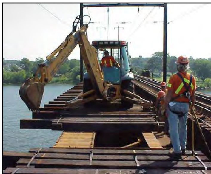
With the help of a backhoe, a Bridge and Building crew sets new ties in position on the Susquehanna River Bridge.
