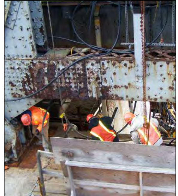
Bridge and Building crews modify the platform used to support bridge control cables during the replacement project.
