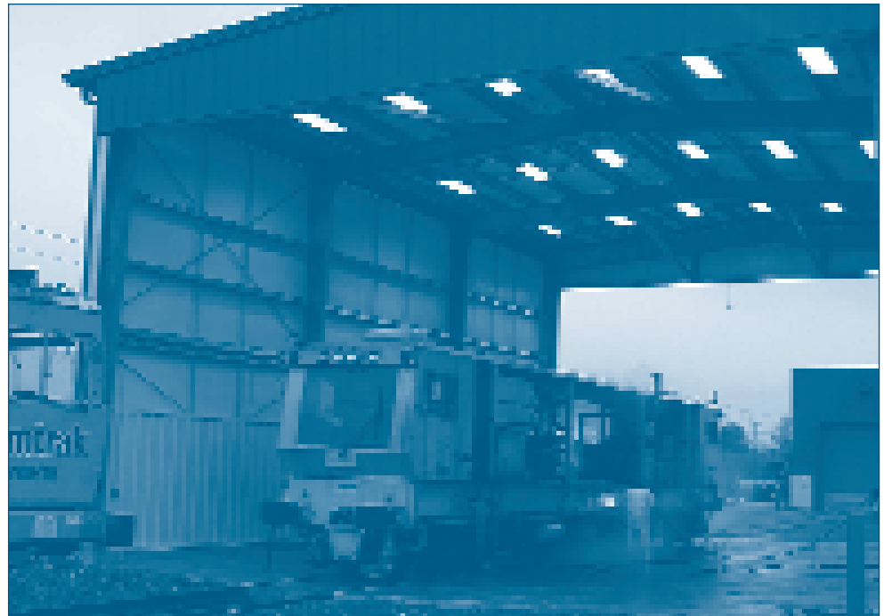
A track stabilizer is cleaned at the new spray wash facility located at the Providence Maintenance-of-Way base. Opened in December to handle large pieces of track equipment and oversized work vehicles used by the Engineering department, the facility enforces stringent pollution controls and is more efficient than its predecessor.
