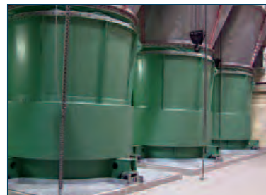
The $470 million Phase I includes rehabbing four ventilation systems and installing a standpipe fire system. These 63-foot tall, 23,300-pound fans are part of the completed system at the North River Weehawken ventilation site.
