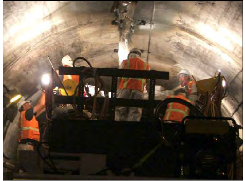
Contractors apply a final coating of a waterproofing compound to the ceiling of one of two East River tunnels in Queens, NY.
