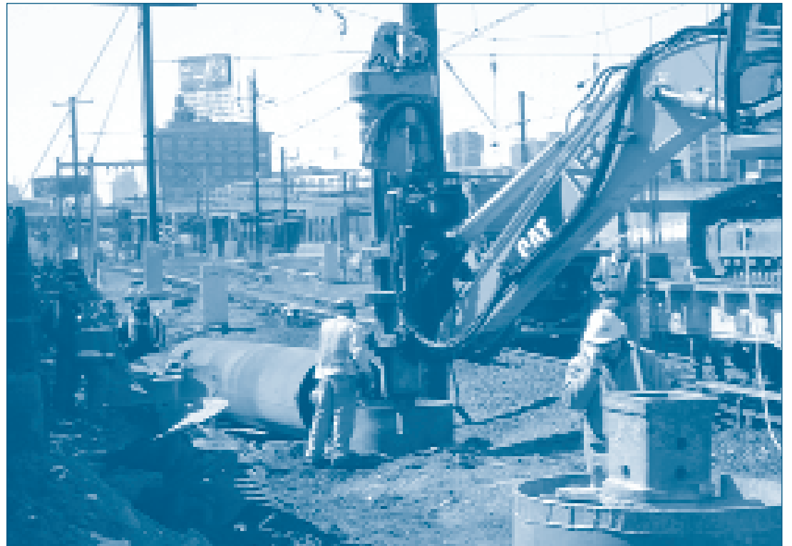
At New York's Sunnyside Yard, new catenary pole foundations are being drilled as work begins to accommodate additional tracks for the East Side Access project. The long-term project between Amtrak, the MTA, Long Island Rail Road and Metro-North will benefit commuter agencies and Amtrak by providing direct access to Grand Central Terminal for LIRR commuters and reduce congestion in the busiest railroad interchange in the country.
