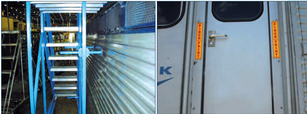
At the Ivy City Maintenance Facility, new, safer scaffolding that locks against the locomotive body replaces an outdated apparatus while train doors are now labeled to identify hazardous pinch points.
