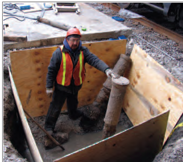
Bridges and Buildings Mechanic Enrique Carpintero excavates and repairs two water leaks off of storage track four at the Chicago Yard. The repair of these and other leaks at the facility has saved the company an estimated $200,000.
