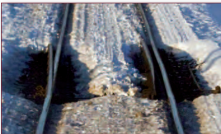
Eliminating snow-packed or frozen switches enables trains in the Midwest to operate continually in and out of the region.
