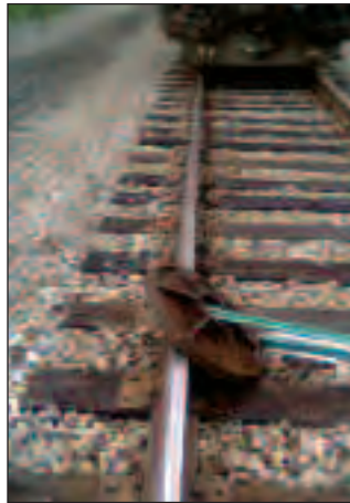
Photo: Kevin Chittenden Above is the obstruction, which included a propane tank and a manhole cover and fence posts wedged across the track near Albany, N.Y.
