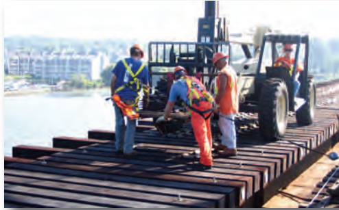
Installation of nearly 50,000 wood ties and timbers is a significant part of Engineering’s FY ’10 capital program.
