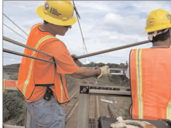
Nearly $30 million is slated to improve Electric Traction capabilities, including renewing 50.5 miles of catenary hardware, installing new insulated power cable and upgrading frequency converters at Metuchen, N.J.
