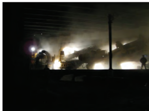
This shoulder cleaner removes ballast along tracks, then sifts it to remove sand, dirt and other materials before dumping it back in place. Starting this spring, over 300 miles of track are undergoing shoulder cleaning to improve drainage and maintain track performance.
