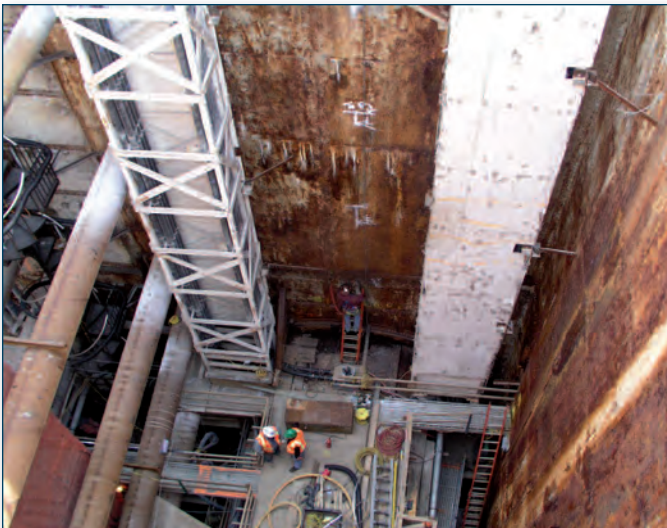
The construction project team gears up to demolish the old structures and all the concrete in the two caissons before fitting out the caissons with new structures that replaced virtually all of the original systems.
