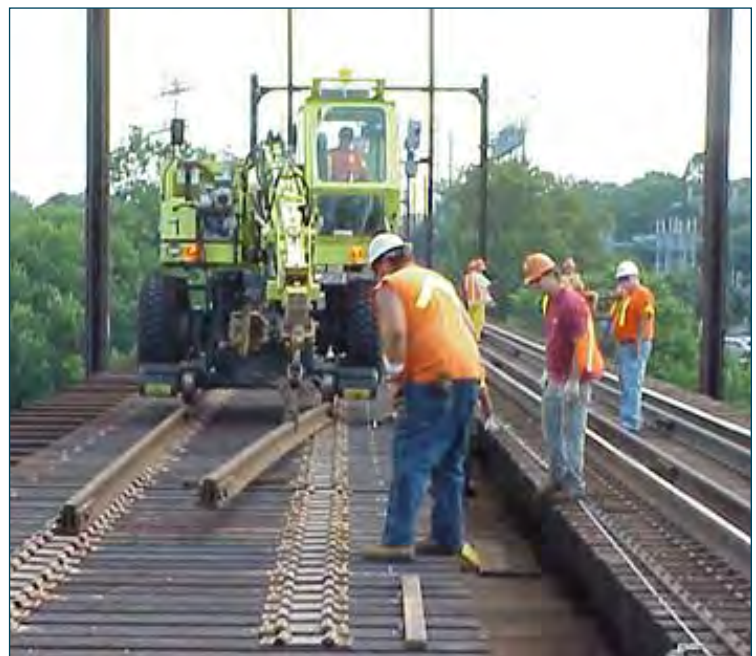
Track department employees put stick rail in new tie plates on top of new ties. The stick rail becomes the inner rail guard when the Continuous Welded Rail is installed.
