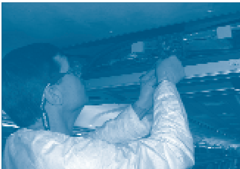
Electrician Anthony Testa installs wiring in the disaster lighting system of cab car 9646.
