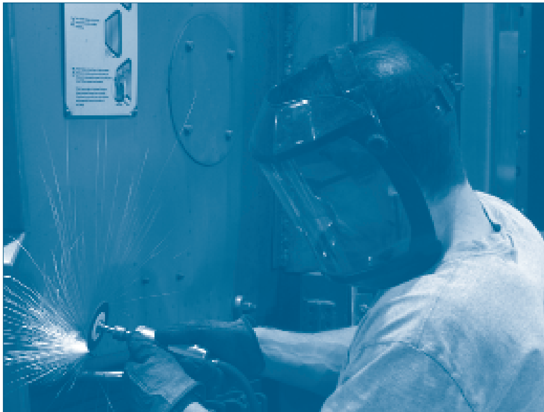
Car Repairman/Welder J. Bruce Carlton installs a grab iron on cab car 9646 at Bear Car Shop. The grab iron is a safety feature used by the crews to hold on to when pulling cables or coupling the train.
