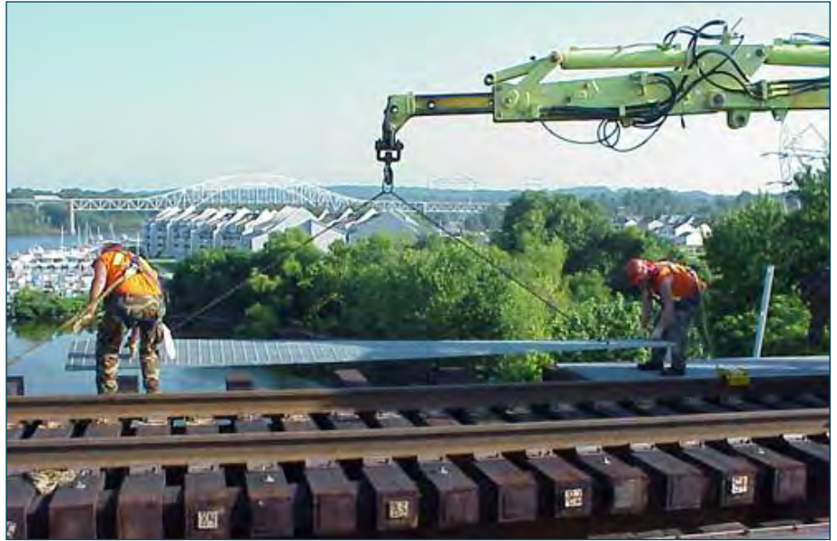
With safety harnesses that are connected to rail trolleys, Bridge and Building employees install grating for a new walkway with the help of a Geismar Crane operated by the Track department.
