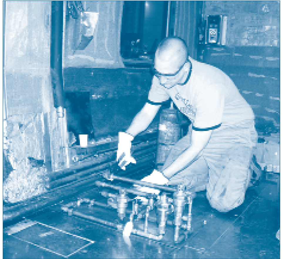
Pipefitter Jon Gedek installs water piping in Superliner I Sleeper Car 32056, scheduled to be released next month.
