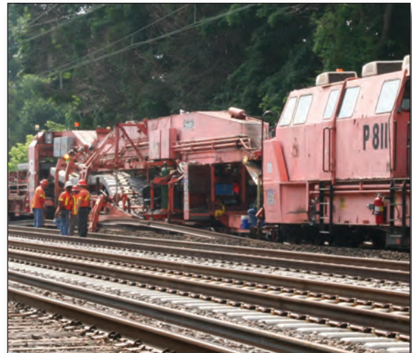
The Track Laying Machine, which installs ties and welded rail, works on the NEC near Wilmington, Del. The TLM is helping replace almost 150,000 ties this year.
