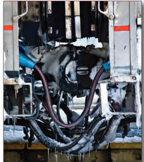
Exposure to the elements causes freezing of air and electrical hoses. However, most components on the Superliners are housed in compartments rather than outside the car body.
