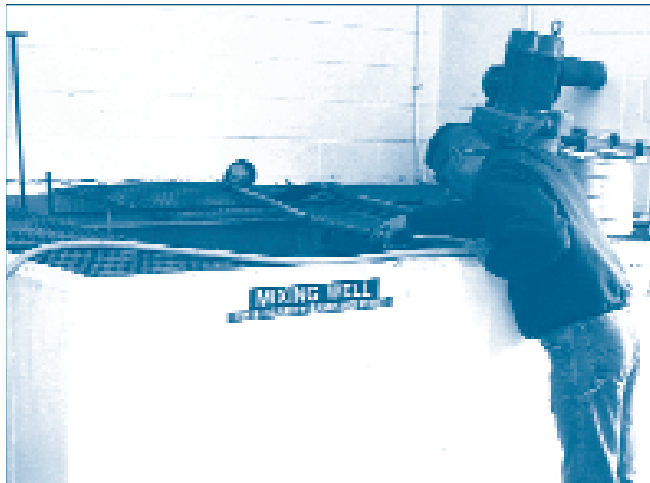
As a wastewater treatment operator, Christopher Lento (currently a Mechanical foreman III) monitors the mixing tank where chemical additions and pH adjustments are made to the wastewater prior to its transfer to the DAF system’s primary treatment tank.
