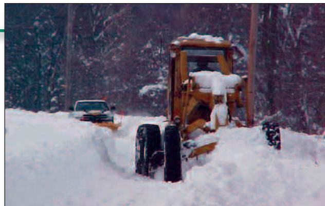
Photo: Andrew Keefe Equipment Operators Don Rivers and Tracy Fowler use a bulldozer and snow plow truck, respectively, to clear a track access road in the Hudson Sub-Division near Albany, N.Y.
