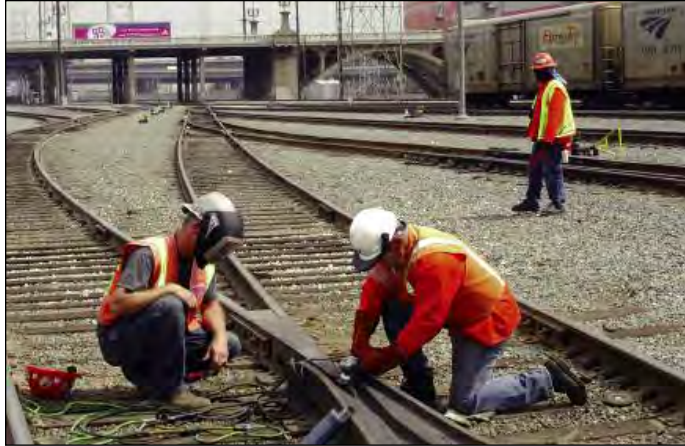
Photo: Abel Hayes Maintenance of Way workers (L. to R.) John Powers, Mark Paguirigan and Reggie Hawkins at the 8th Street Yard in Los Angeles perform maintenance on a switch frog.
