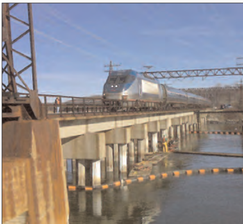
Work is underway on the Pelham Bay Bridge on the initial concrete chipping. When completed in October, the bridge will have repaired piers, piles, abutments and foundations that support the tracks, transmission lines and catenary wires.
