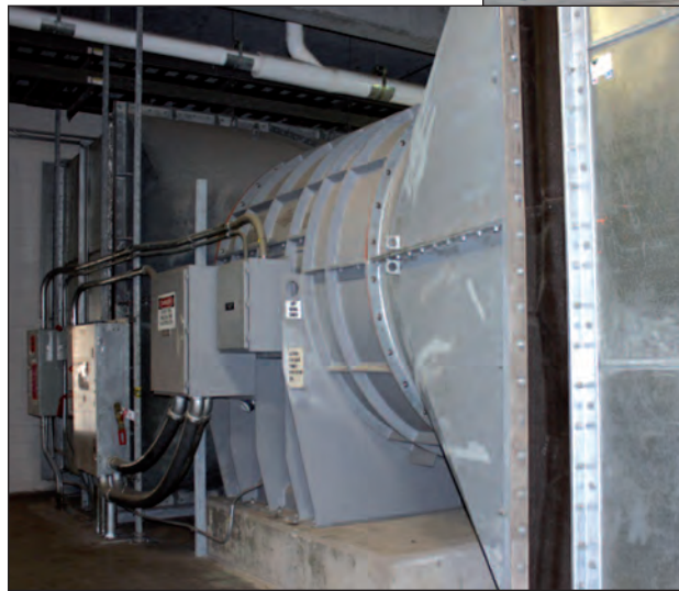
The Long Island City Facility (top right) houses one of three completed ventilation systems (shown above). The fourth ventilation system at First Avenue is slated for completion in Feb. 2011.
