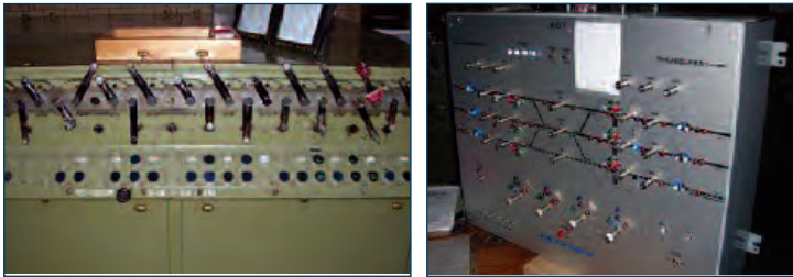
The old lever system (left) to control signals and switches along the Keystone Line between the State and Roy interlockings has been replaced by a modernized push-button system (right).
