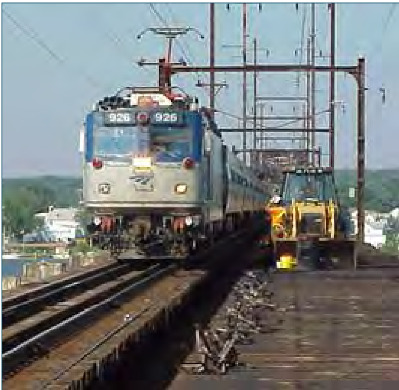
Bridge and Building employees pause the installation of new ties on Track 3 as a train crosses the Susquehanna Bridge last summer.
