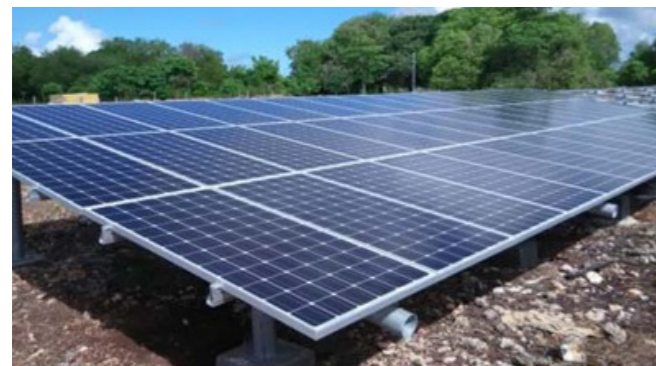
Solar Power Plant, Selayar Islands Regency, South Sulawesi
