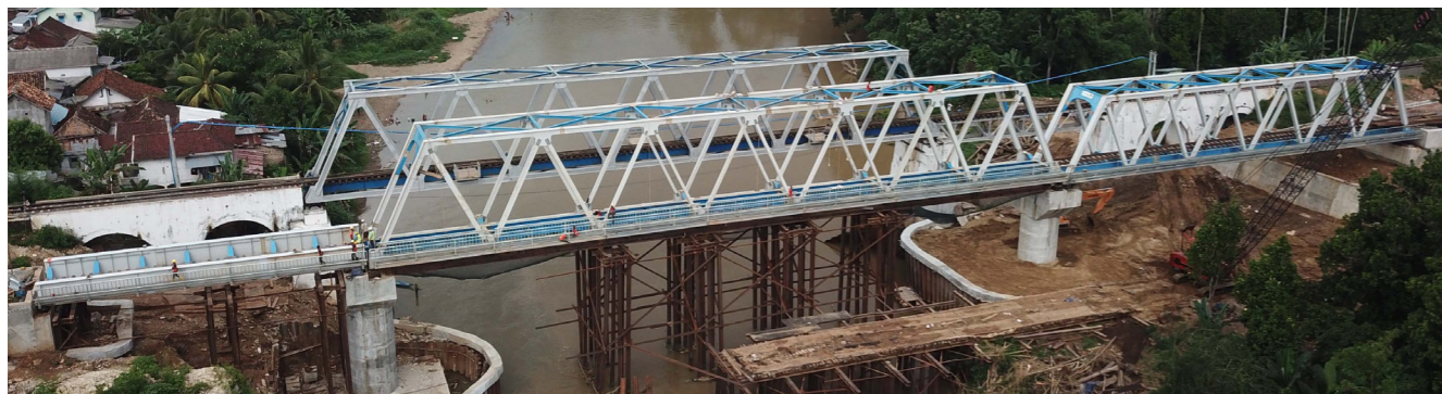
Construction of the Martapura-Baturaja section of the Trans Sumatra Railway, South Sumatra.
