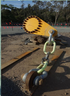
HDD completed. Pipe inlet at Orbest plant. Now connected to subsea pipe.
