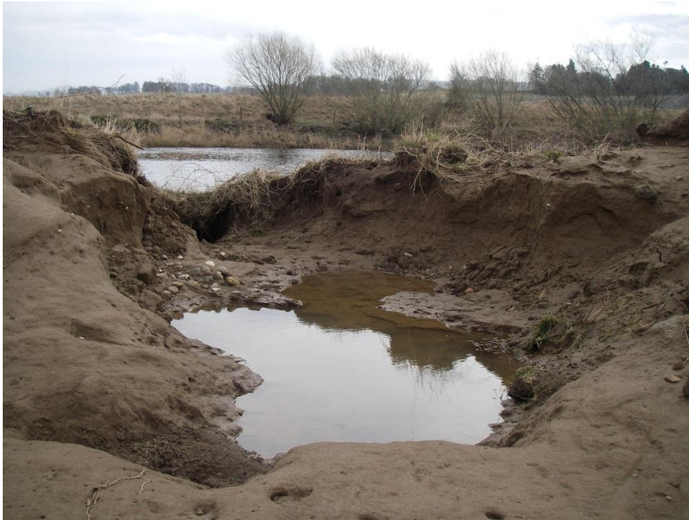
Figure 30. Flood bank breach
