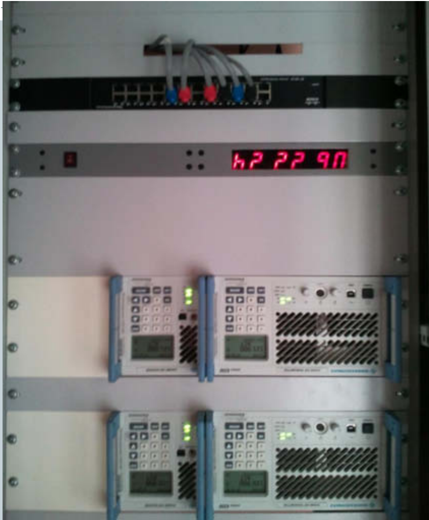
VHF transmitter and receiver
