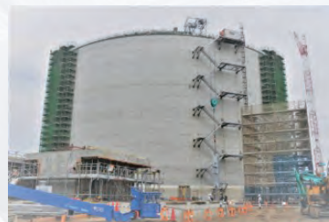
Building an LNG tank, the largest of its kind in Japan, on the premises of Ehime Works
