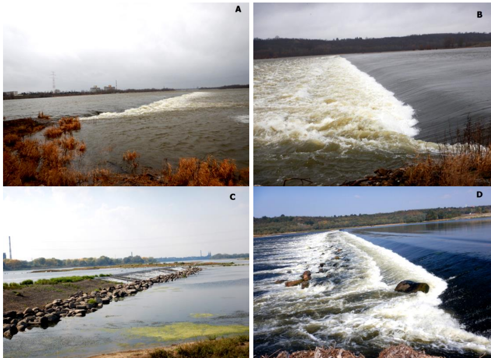
Figure 2.3.12. The auxiliary dam: right (A) and left (B) side, Jan 2017, flow 1,264m 3 /s; right (C) and left (D) side, Sept 2016, flow 407m 3 /s.
