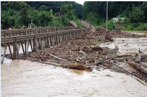
This metal bridge across the Khon River that links the main road leading from the Luang Namtha provincial capital to Nalae district is now impassable. —Photo Pathedao Lao
