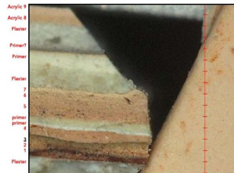
Stratigraphy / Analysis of the paint layers conducted during the 2009 interior restoration of the La Roche House – Dining room
