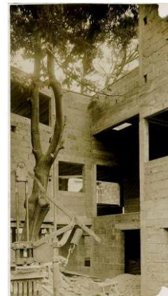
Construction site of the La Roche House, entrance hall and bay window, 1924 (FLC L2-12-22)
