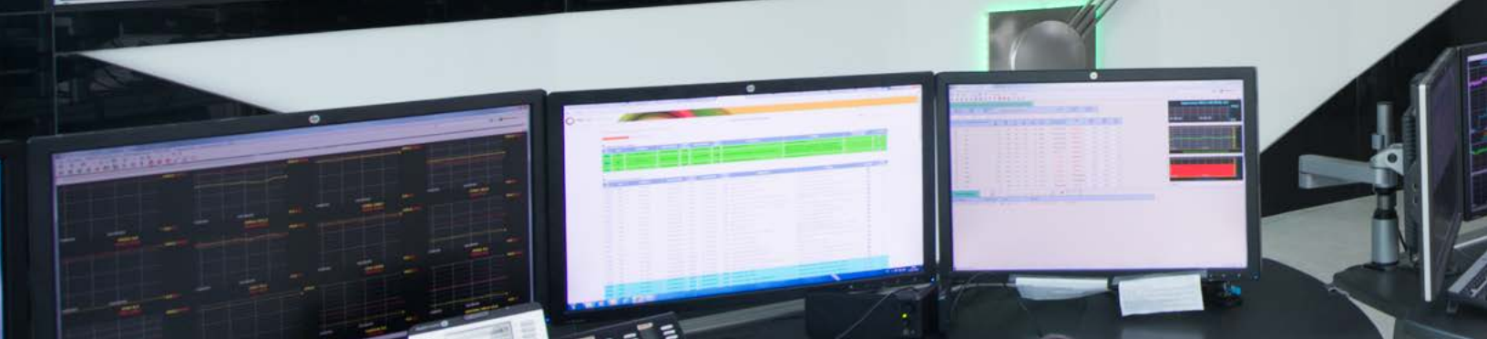
Sala de Control, CDEC-SING
