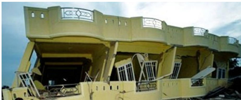
Figure 5.4 Pancake collapse of reinforced building in Padang (from Reuter)
