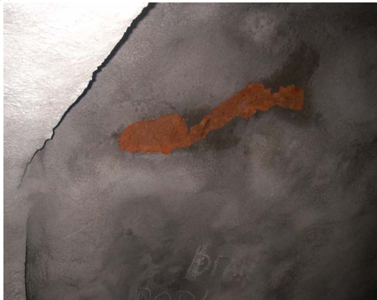
(b) Spalling at Location 3
