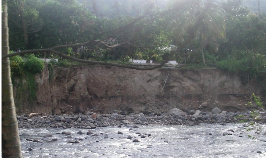
(a) Embankment failure at Sumpur Village (the nearest site to the epicenter)
