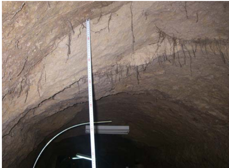
(a) Roof falls
