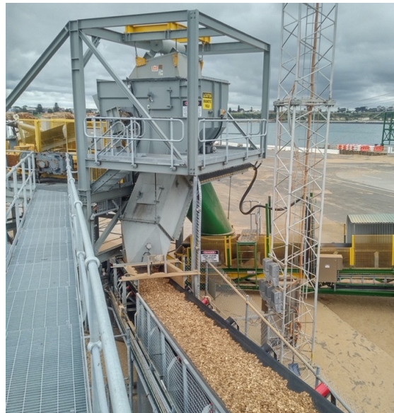
Figure 22 Case C - Re-Chipper Station
