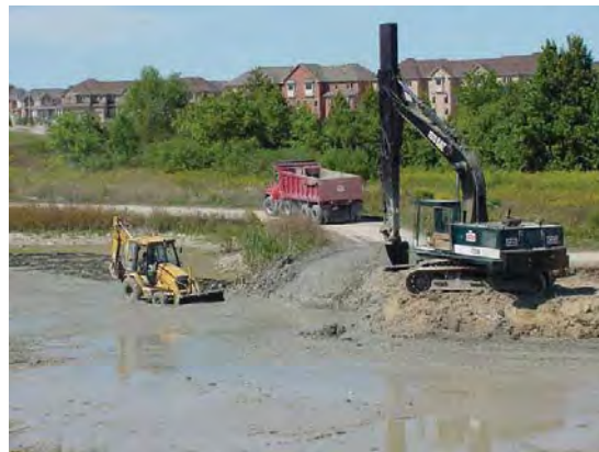
Sediment removal is part of regular stormwater management facility maintenance (Photo credit: Town of Richmond Hill)
