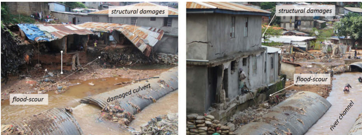
FIGURE 14: Flood Damage in Culvert
