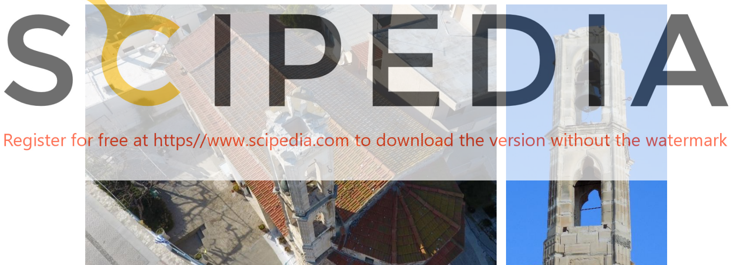
Figure 6: Bell tower of Saint John's church in Psevdas village after the earthquake (photos taken in February 2017)
