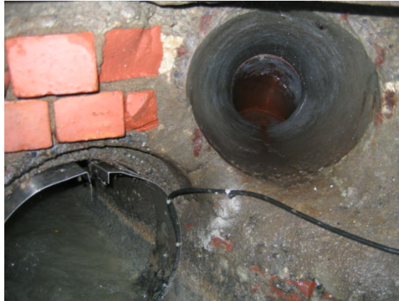
Figure 4: High level overflow pipe between sewer and stormwater in Wellington city wastewater manhole.
