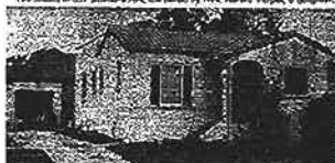
This house at 3077 Bonadira St., on route of new freeway, is being demolished.
