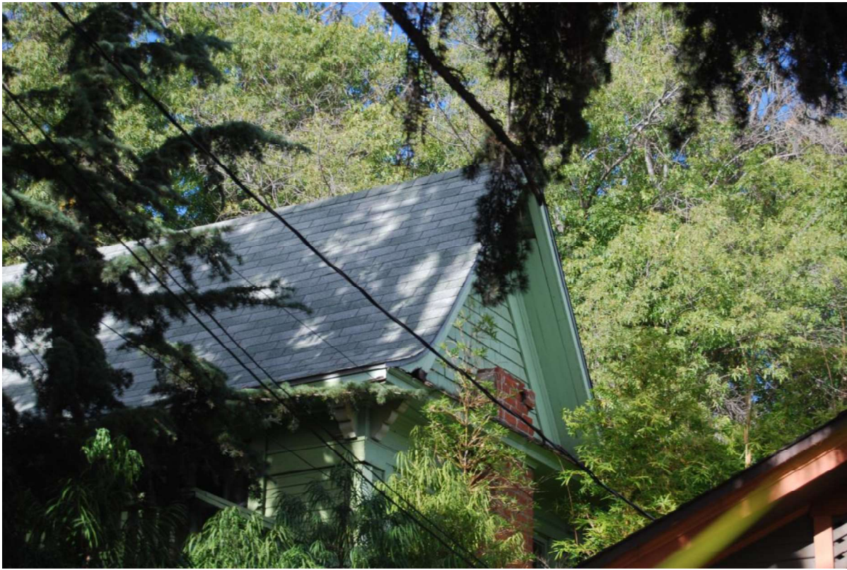
Queen of Elysian Heights, earthquake damaged chimney, 1553 W. Ewing Avenue, November 22, 2021 (Photo by Charles J. Fisher)
