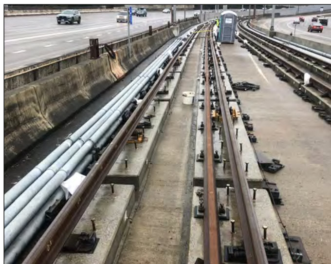
New track plinth fixation inserts installed near the east approach to floating bridge
