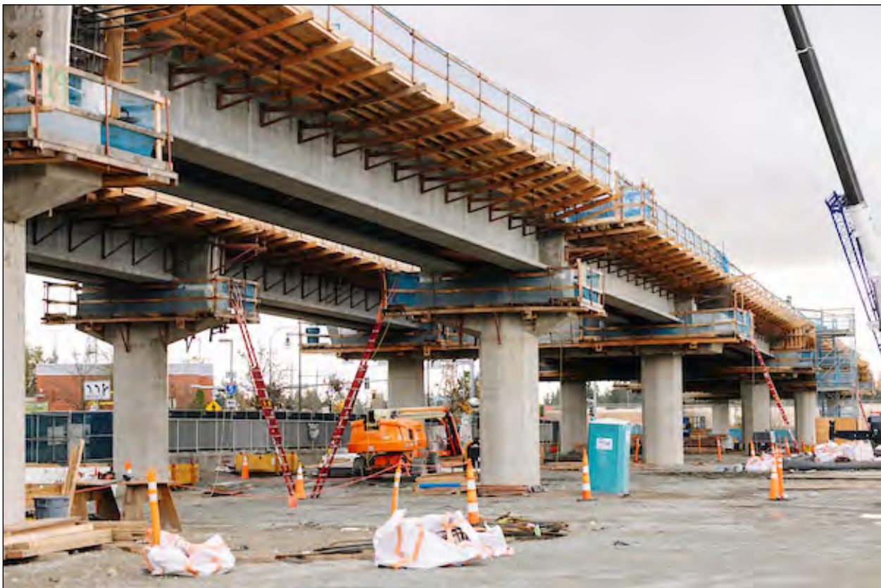
Federal Way Transit Center Station construction progress December 2, 2021. Federal Way Link Extension
