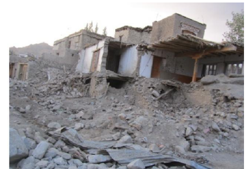
This photo showing the damage in Saboo village due to the 2010 Cloud Burst (Photo taken by author immediately after the event).
