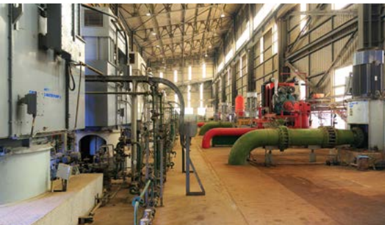
The dimineralized processing plant
