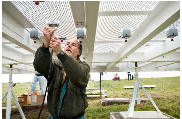
NOAA electronics engineer Tom Ayers installs equipment for an atmospheric river observatory in Bodega Bay, CA. (Credit: California Department of Water Resources)
