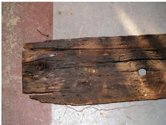
Figure 7 - View of an element that has splintered
