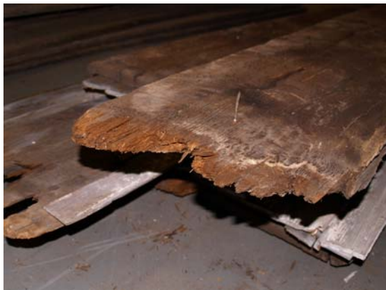
Figure 3 - View of an element that has rotted, resulting in partial loss
