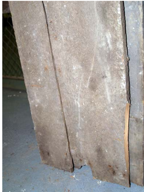
Figure 6 - View of an element that has cracked
