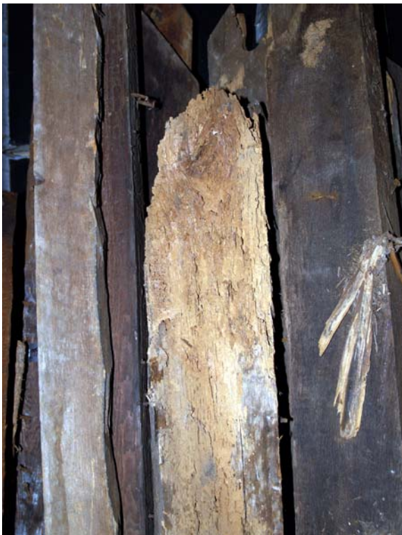
Figure 8 - View of an element that has suffered from insect damage
