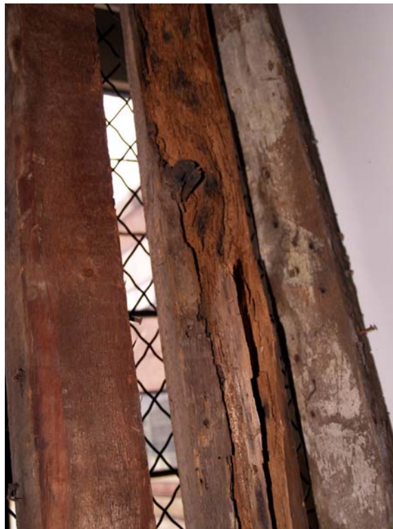
Figure 9 - View of an element that has suffered from insect damage
