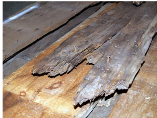
Figure 4 - View of an element that has severely rotted, resulting in cracking and partial loss
