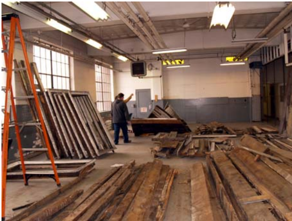
Figure 1 - View of the garage space at 11 Stickney Avenue where the assessment was performed
