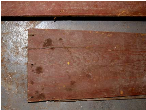
Figure 5 - View of an element that has cracked
