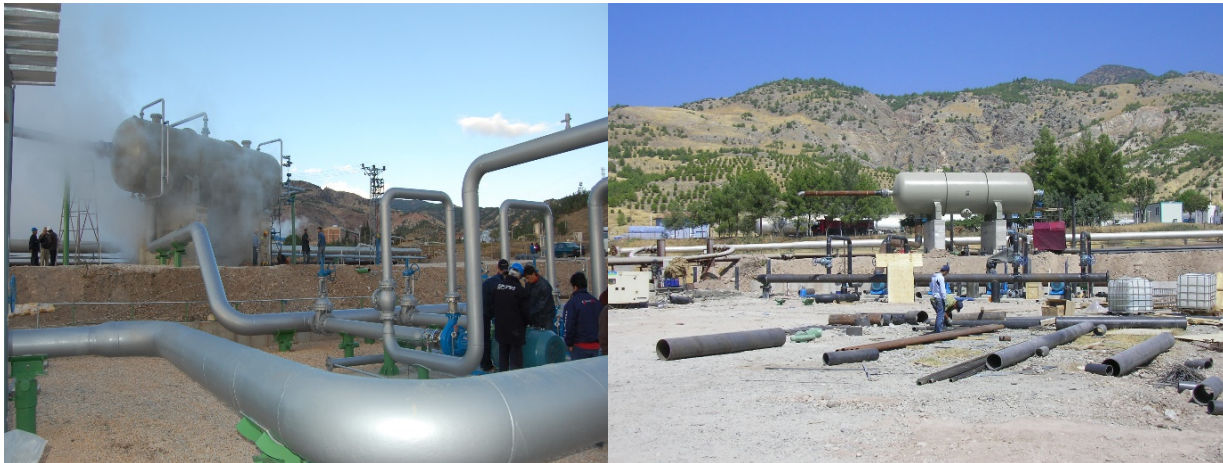
Figure 4: First reinjection pump station in Kızıldere field.
