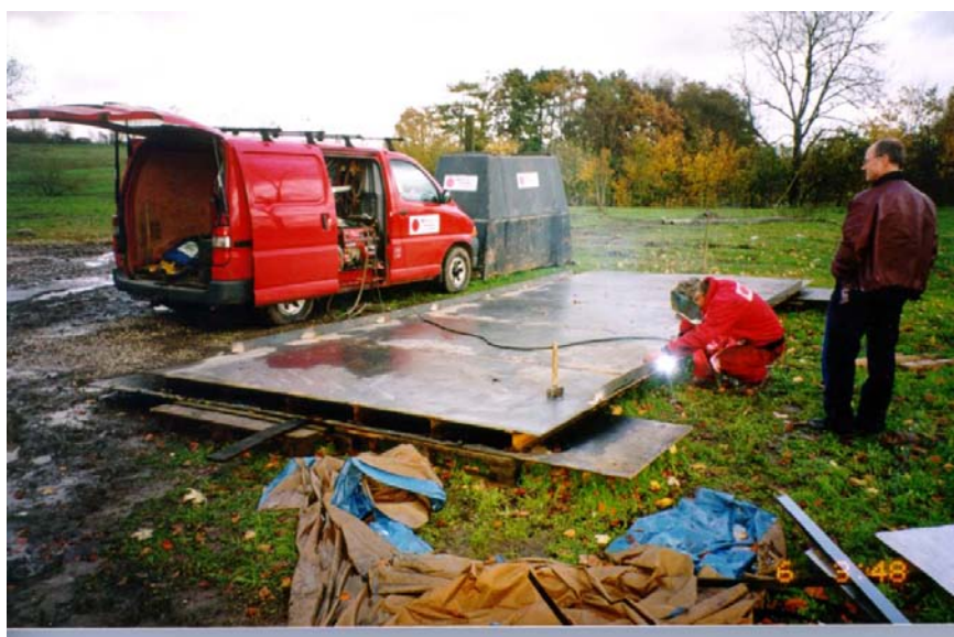
Welding the bridge. The bridge is moveable and only lies on the two plates seen beneath each end. After positioning the bridge surface is covered with 5 cm of soil.
