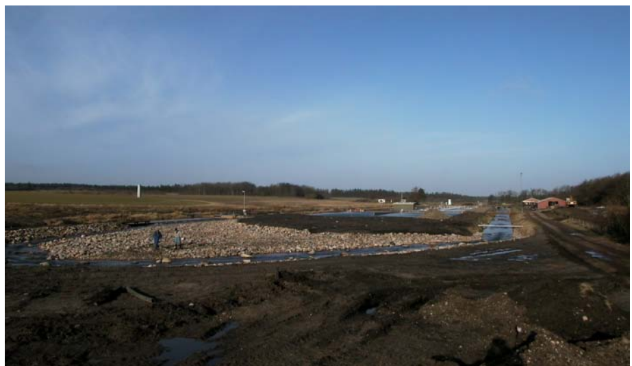
The newly established fish pass at Gryde Fish Farm
