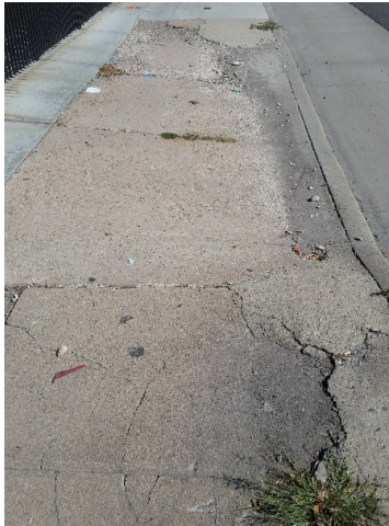
Colfax Ave east of Utica Cracked and uneven surface
