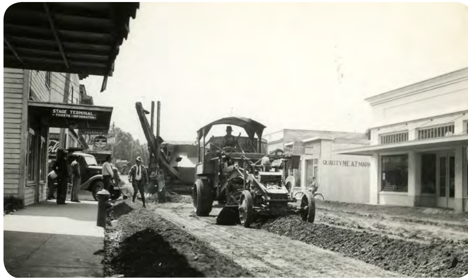
left 1928 toad construction in Poulsbo, possibly current SR 305. Source: Washington State Archives.
