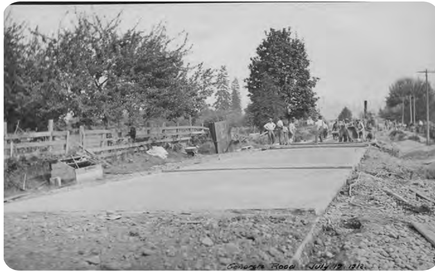
right Building state's first concrete road - possibly portion of SR 507 in Lewis County. June 19, 1912. Source: Washington State Department of Transportation.
