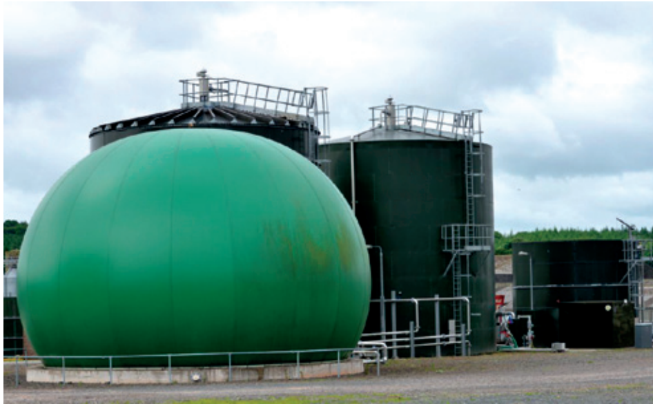
An on-farm anaerobic digester plant showing the gas storage tank and digesters 1
