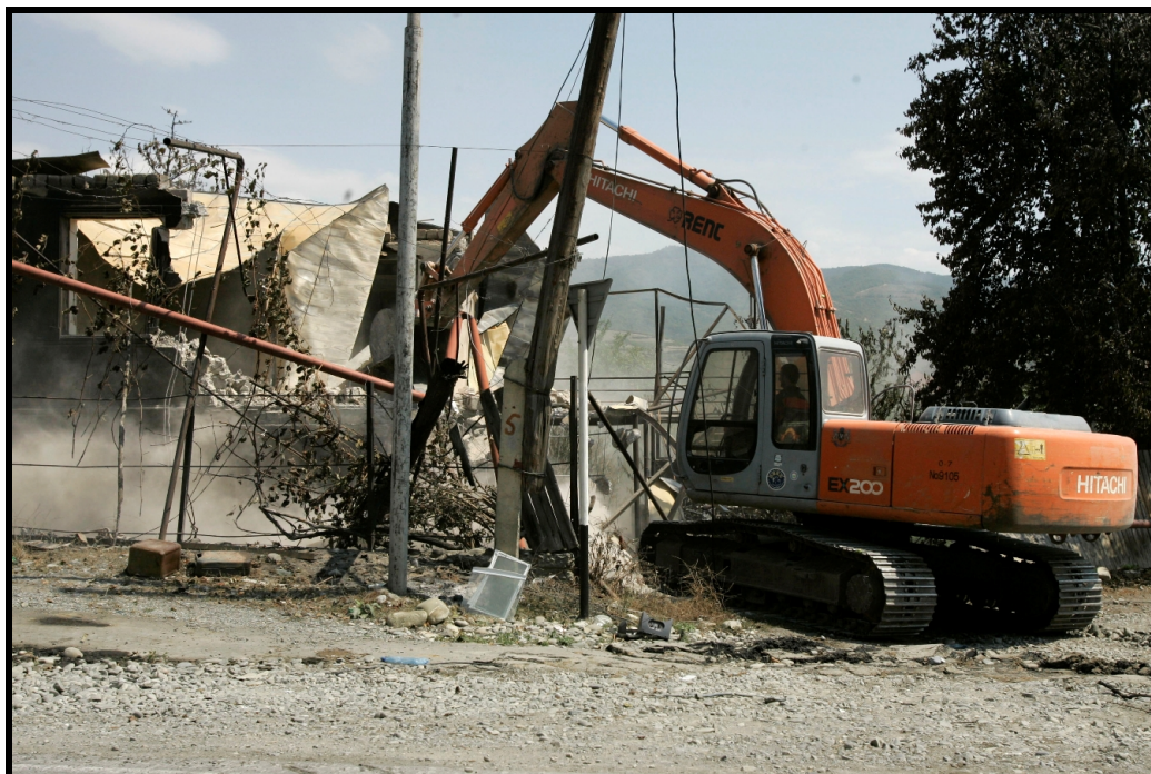
Photograph 3.6 - Excavator tears down a destroyed house in Achabeti (22 August 2008). (AP Photo/Dmitry Lovetsky)
