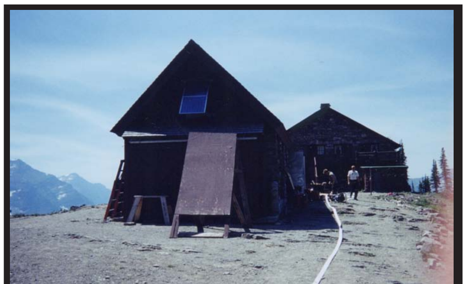
Trail crew deploying hose at Granite Park Chalet on July 21.. (John Hagen Photo)
