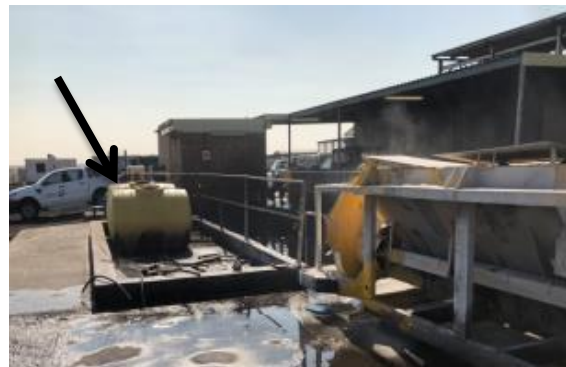
Photograph 2-8: Oil skimmers at wash bay
