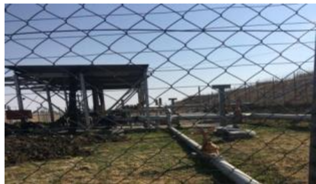
Photograph 2-4: Existing pump station
